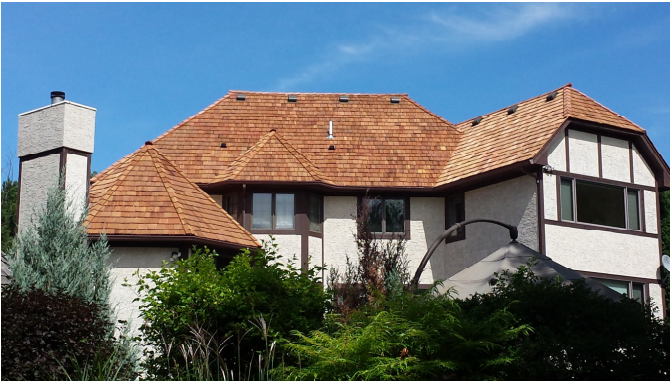
Cedar shake roof repair completed by Veterans Integrity Exteriors following storm damage in Eden Prairie, Minnesota
